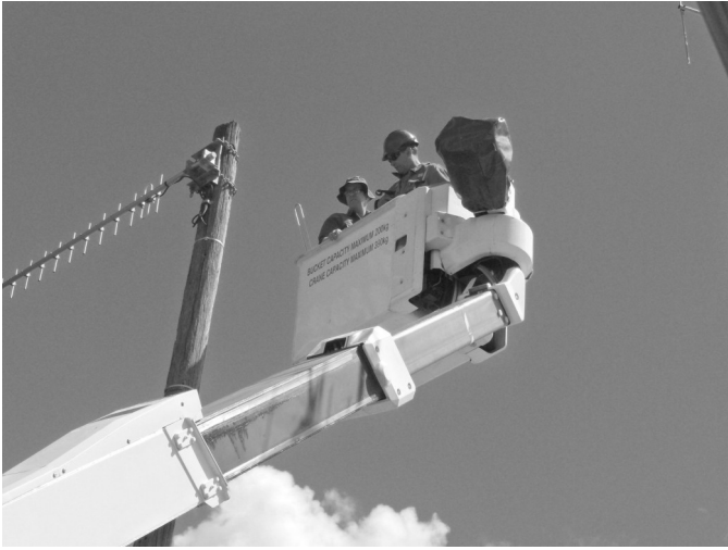
Ewan Mason and Dave Ponton fixing the new FM aerial onto the mast at Burn Radio Station. The low powered frequency is free to not-for-profit radio stations and will broadcast to a 4km radius, allowing visitors searching FM in their vehicles to tune in to local content (and another option for locals who perhaps haven't been able to get AM on their stereos at home).
