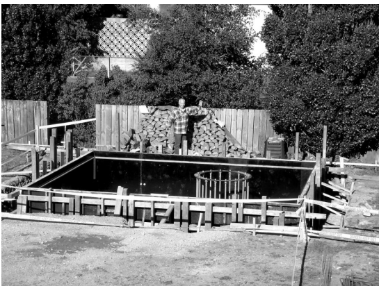
Above - Bill McIntyre from The Old Post Office Backpackers gives us an idea of the scale of the construction.
