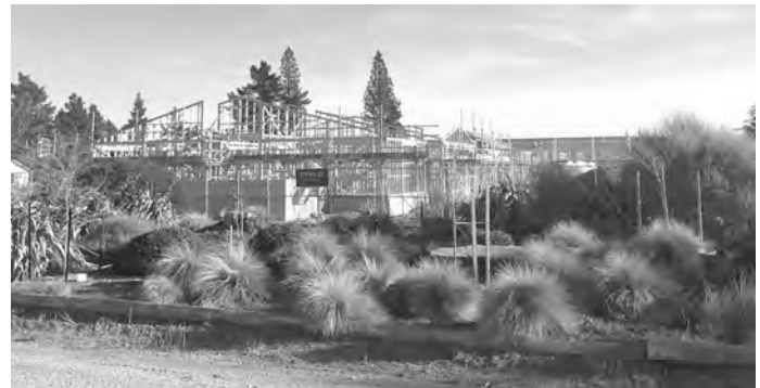
The rapidly progressing Maniototo hospital and rest home re-build is now beginning to make its mark on the Ranfurly skyline.
